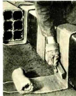
Experimental conduit joints are made with a plastic cement mortar saturated bandage.
