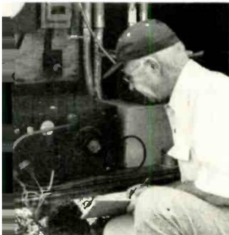
Bill records data from a voltmeter on a test of a buried high voltage cable.
