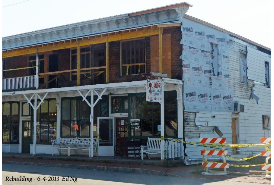
A fire in an upstairs apartment damaged the building that houses Taylor's Ice Cream Parlor and other businesses in Chester on Friday. For a photo gallery and video, go to DailyRecord.com . APRIL 9, 2013 CAP/STAFF PHOTOGRAPHER Daily Record March 9, 2013 Fire damages iconic building.
