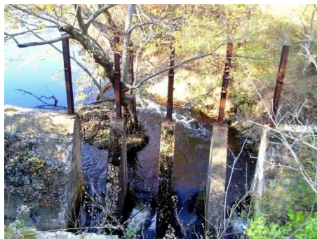
Remnants of the dam 7/7/2021
