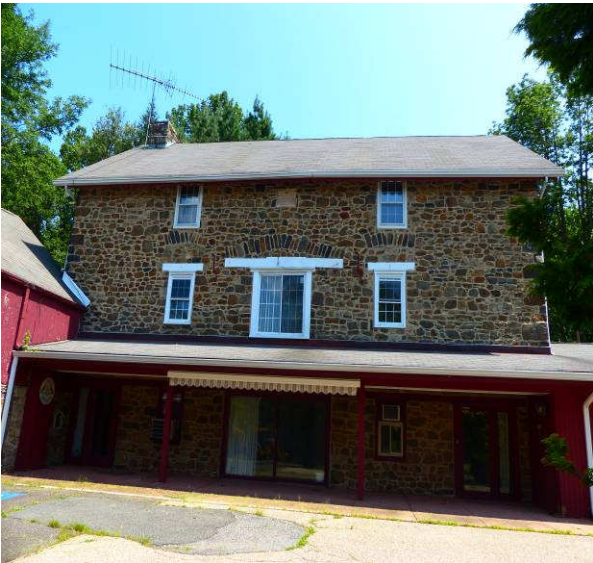
Southwest or front side of the barn The stone front wall and the pent roof or roof overhang above the doors, are indicative of the English Lake District type barn. The curved window arches and metal S anchors add an "air of refinement".
