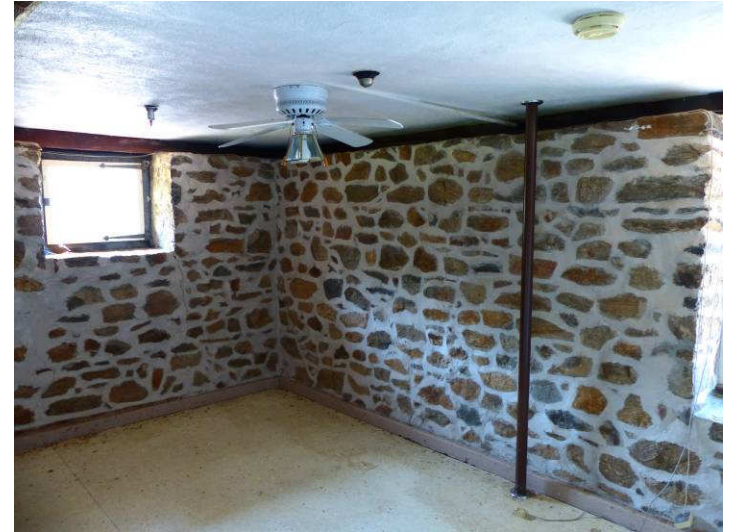
Second floor room-could have been an office The interior was much altered by the Bodens.
